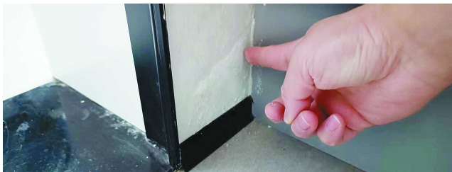
一楼卫生间门边墙角渗漏
